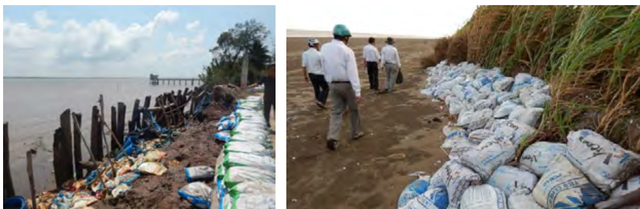
Fig. 43. Emergency repair of sea-dykes in Soc Trang and Ben Tre using sandbags. The crucial point for emergency repairs using sandbags is the method of stapling.
