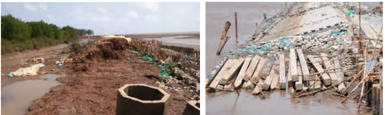
Fig. 42. Sea-dyke-like embankments in front of the mangrove forest in the East Sea (after dyke breach) and West Sea (under construction in 2017). This practice is strongly discouraged since it will diminish the ecological and economic value of the mangrove forest and requires immense investment and maintenance costs. Alternatives are breakwaters as described in section II.
