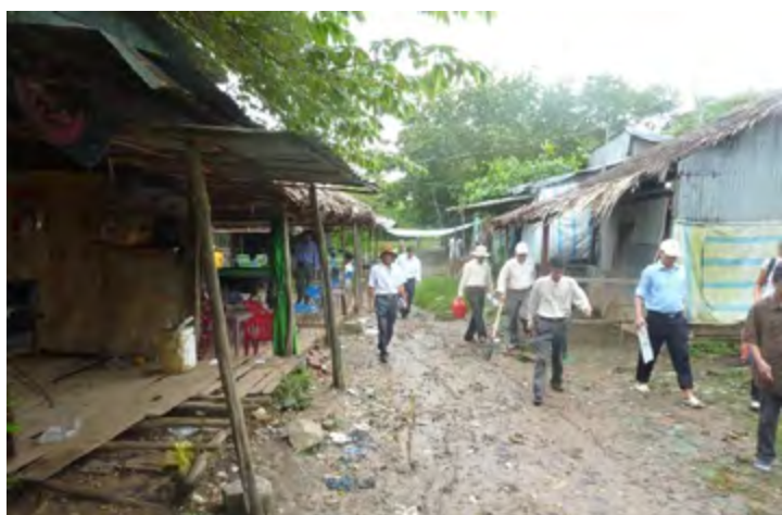
Fig. 8d. Earthen sea-dyke along the West Sea coast of the Mekong Delta. This sea-dyke will be strengthened in the near future. An unsolved problem are the settlements on the dyke crown or berm along several stretches particularly at the West Sea. The site of the settlements are offering some safety for people living on resources in the dyke foreland and nearshore but makes the dyke itself very vulnerable.
