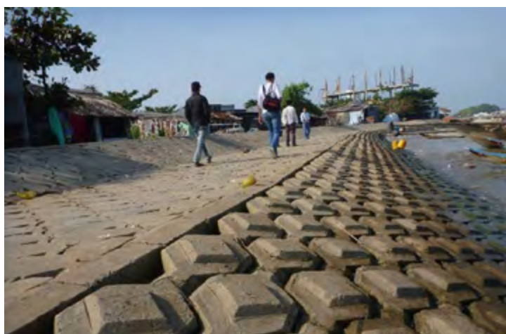
Fig. 8c. Heavily armoured sea-dyke along the West Sea coast in Ca Mau province using interlocked slabs. Armouring or revetment of dykes is expensive and critical issues were found during the field studies for the CPMD concerning missing filter layers under the slabs and insufficient dyke toe protection at some sites.
