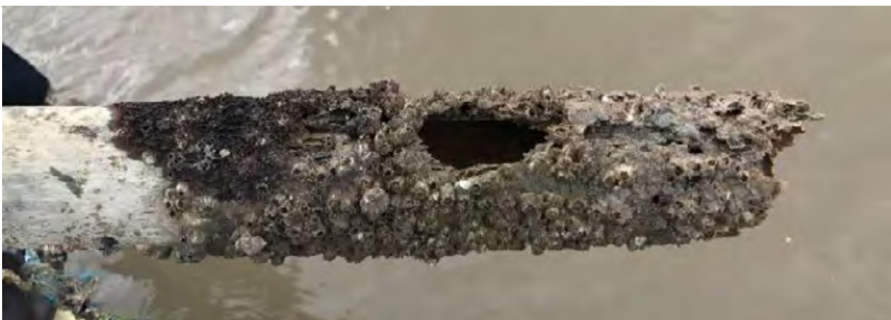
Fig. 56. Bamboo pole destroyed by shipworms. Shipworms attach as free-swimming (pelagic) larvae to the wood surface (all kind of wood) and burrow holes and cavities deep into the wood while growing. The visible barnacles are harmless and do not burrow into the wood.
