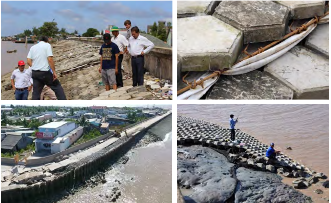
Fig. 41. Concrete sea-dyke revetment at Ganh Hao (Bac Lieu) using interlocked slab-tiles as an example. After high storm surge in 2016, the structure failed. The thickness of current concrete revetment in the case in Ganh Hao might not be sufficient. High waves caused pressure and uplift of the concrete blocks. A milder outer slope is recommended in order to reduce wave run-up and overtopping. Since the blocks seen to be placed directly on clay soil and a geotextile, high uplift pressures can be expected in case of breaking waves. A gravel layer between blocks and geotextile as well as a sandy subsoil in the vicinity of the revetment is recommended. Natural riprap (using large stones) at the dyke toe are rougher than concrete blocks and therefore are expected to reduce wave-run-up as well as overtopping significantly.
