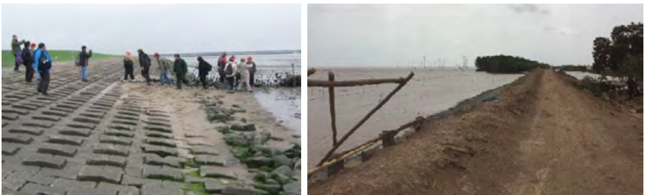
Fig. 39. Left: Typical sea-dyke profile of exposed dyke at the North Sea coast in Germany. The seawards slope of the armoured dyke berm is very mild and even milder close to the dyke toe. The reason is to reduce any damaging wave reflection by water waves with long periods. Protruding interlocked concrete slabs are considered to reduce wave run-up. Water reflection leads to scouring in front of the sea-dyke. The salt marshes in the dyke foreland are typical for temperate zones while mangrove ecosystems are confined to tropical and sub-tropical zones. Right: Sea-dyke at the West Sea (Ca Mau) and East Sea (Soc Trang) with typical maintenance roads on the crest or on the landwards berm (right). Source: Frank Thorenz
