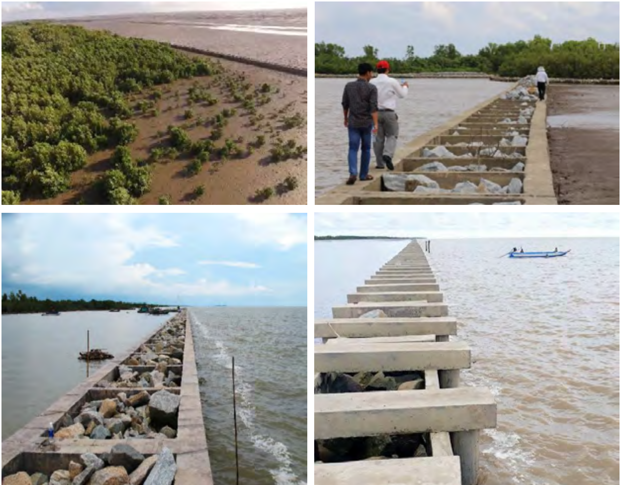
Fig. 11. Detached riprap pillar breakwater along the West Sea coast of Ca Mau. The version below right is the most recent, using larger blocks of stones and partly retractable parts.
