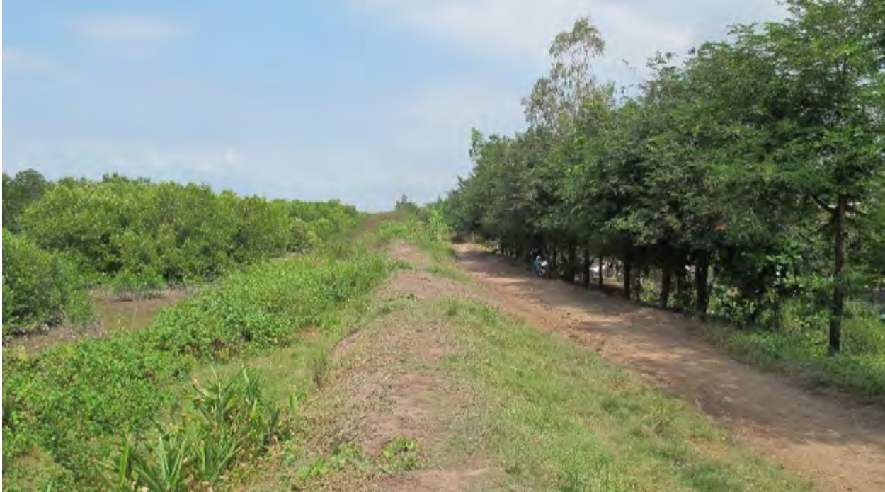
Fig. 8a. Earthen sea-dyke along the West Sea coast of the Mekong Delta. There is still mangrove forest seawards (in the photo left side) protecting the dyke from direct wave impact. The maintenance road for light motor vehicles is next to the dyke crown. However, the dyke is not high enough to protect for flooding and the berm seawards is very steep which makes the dyke vulnerable and leads to unwanted wave reflection. More detail is provided in the chapter on guidance for coastal protection works. Source: Stefan Groenewold
